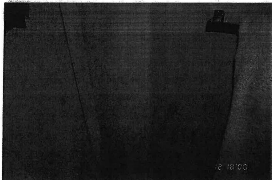
Hole Lower Higdon Bathroom 80087(a)
